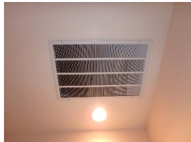
Return Air Grill in Hallway
