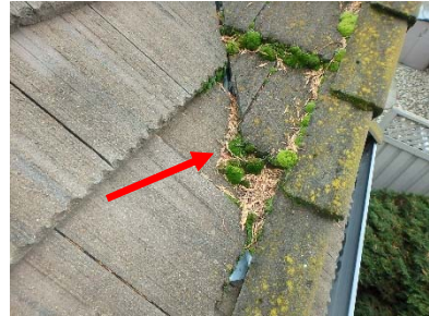
Example – Debris in Valley
