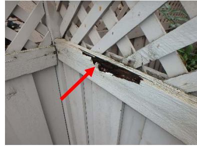
Example – Deteriorated Fencing
