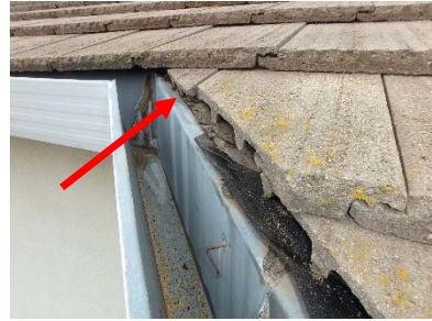
Deteriorated Roofing Paper
