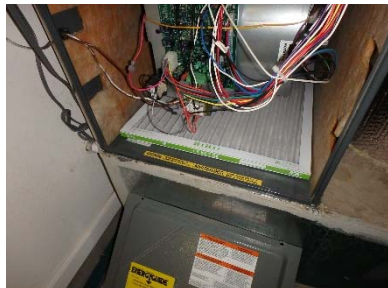
Air Filter Inside Furnace Cabinet
