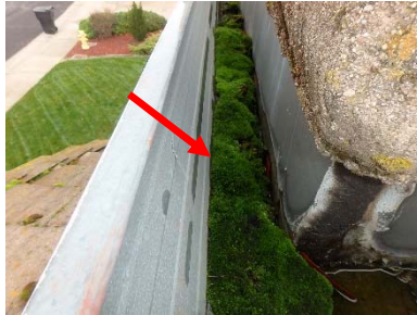
Example – Debris in Gutter
