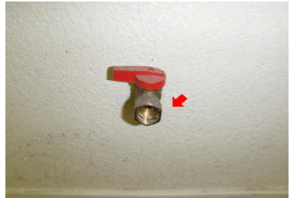
Gas Valve in Laundry Room
